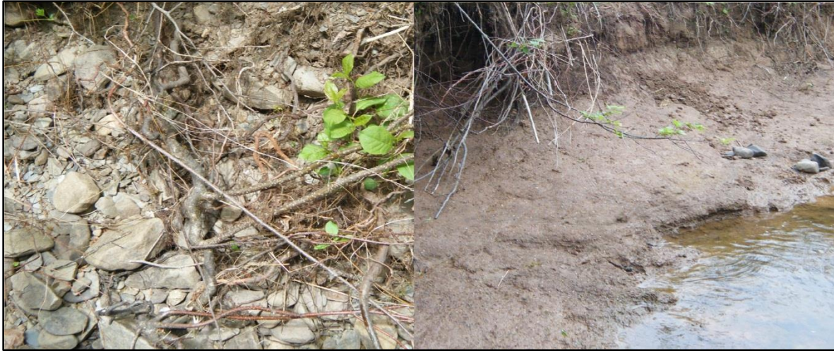
Figure 18 - Stable rocky bank and actively eroding bank
