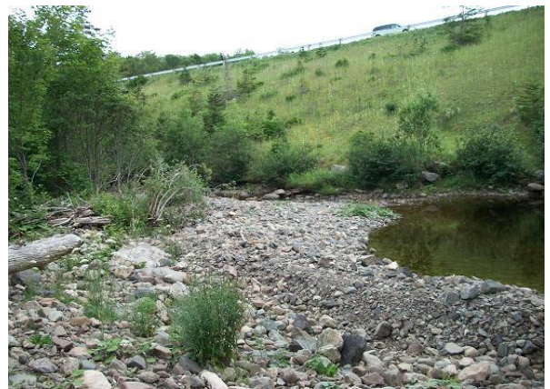
Fig 4 Material scoured out of the plunge pool had been deposited in the channel, blocking water flow
