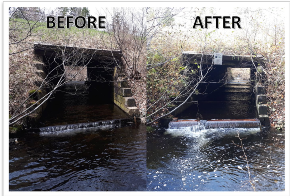
Figure 1: An example of a culvert retro-fit fish passage improvement that utilized an outflow chute and baffles to slow water velocities and increase depth.
